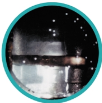
Figure 6-4. More than 60 seconds after start-up, oil level is well below normal operating levels—a condition that is an important factor in compressor bearing wear.
